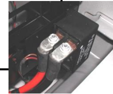
Mount Cut-Off relay inside driver seat pedestal
