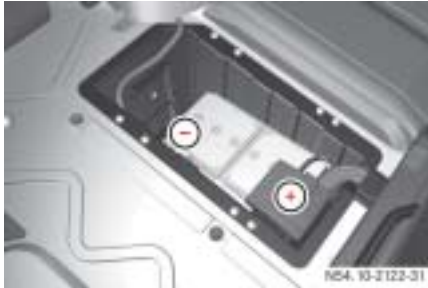
Starter battery in the driver's footwell
